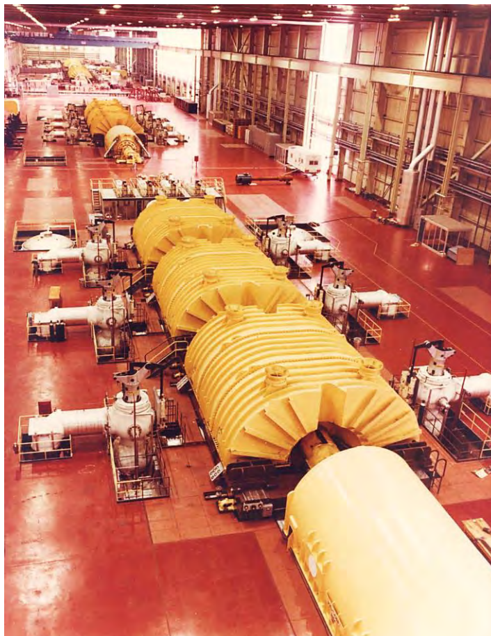
Fig.205 Bruce A turbine hall
