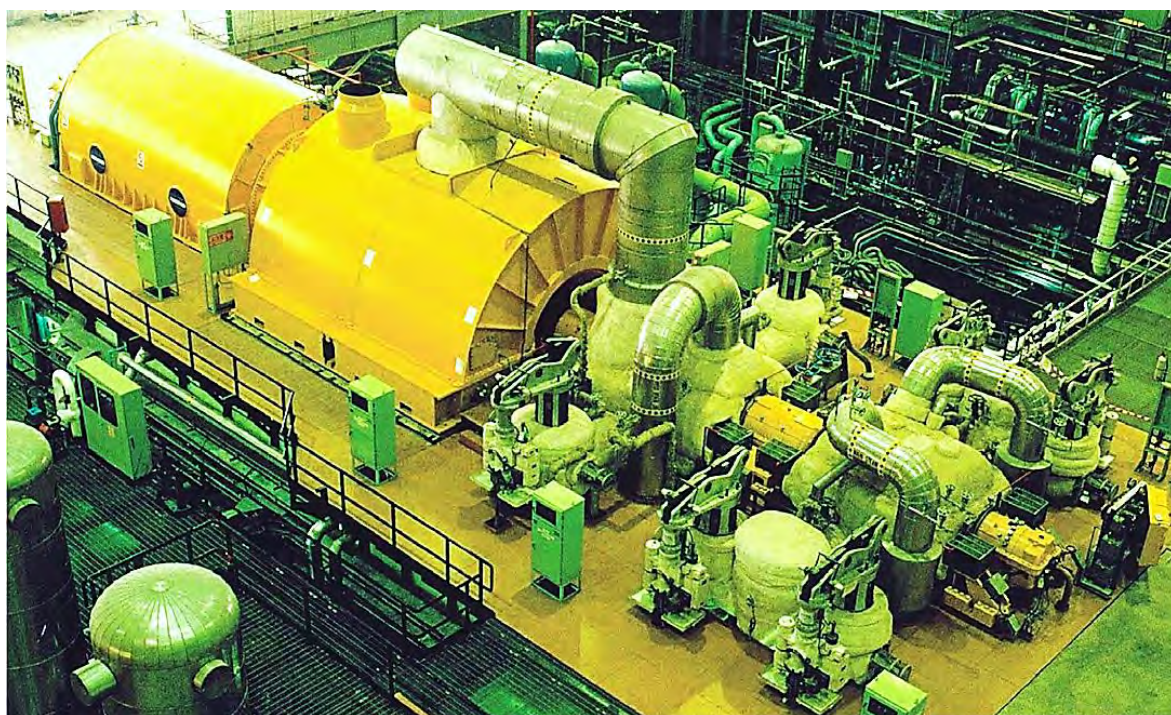
Fig.230 One of the units in Pulau Seraya stage III turbine hall before fitting the acoustic covers
