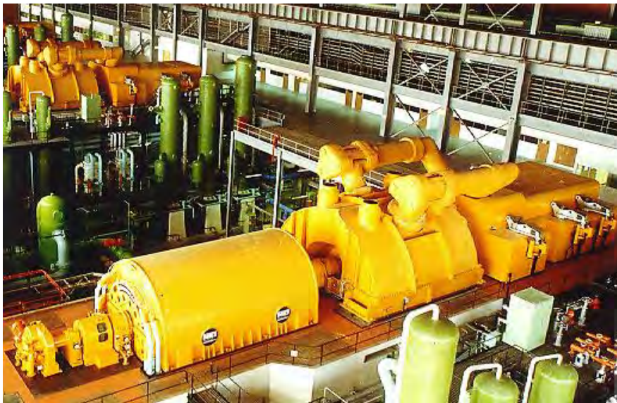
Fig.216 Pulau Seraya stage I turbine hall
