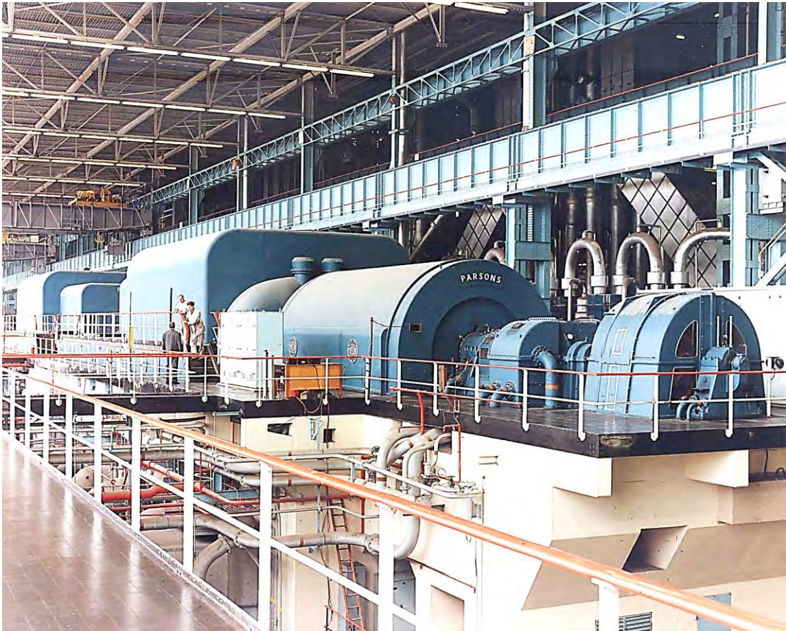
Fig.158 Thorpe Marsh turbine hall showing Unit 1. The two shaft trains were arranged in line with each other, not side-by-side as at other cross-compound stations.
