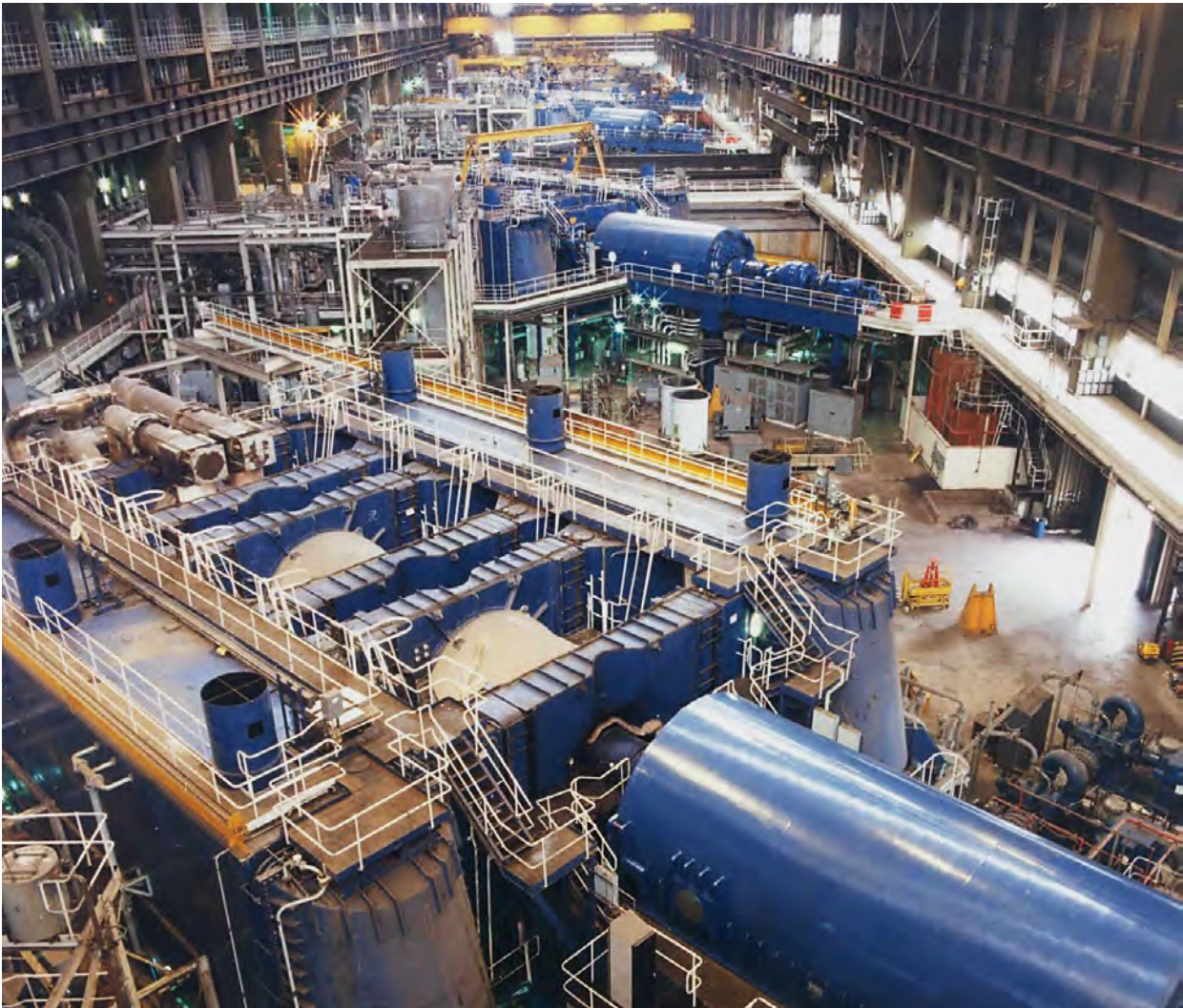
Fig.185 Six 660 MW TG sets installed in Drax
