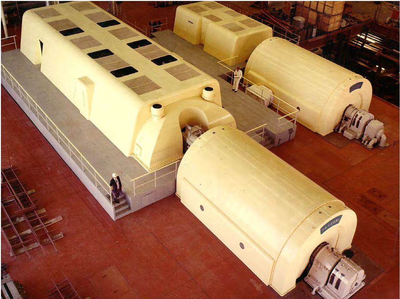
Fig.146 Lakeview Unit 1 installed at the station – A line on the right and B line on the left
